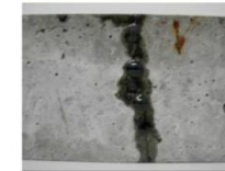
c) Crack repaired in the bottom of Specimen
