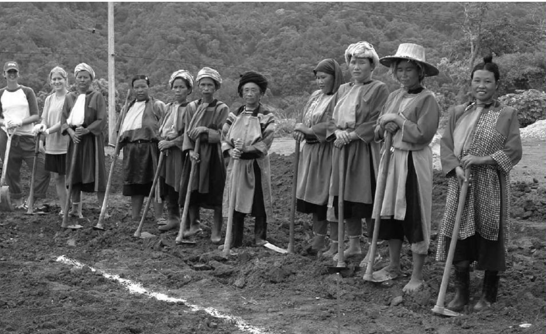
University of Maryland civil engineering students work with women from a mountain village in Thailand to build a wastewater system for a health clinic.
